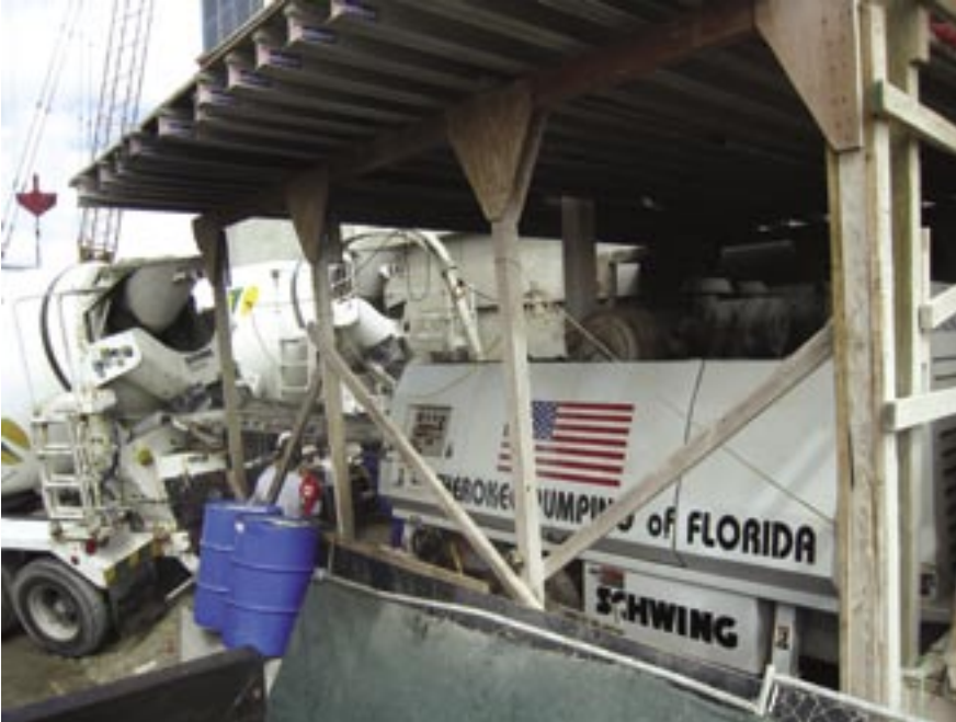
Schwing BP 8800 has broken many high-rise pumping records and will take it to the top on the tallest condo in Miami.
