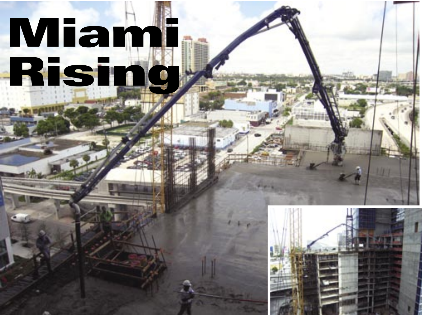
A second 39-meter separate placing boom is working on the parking structure.
